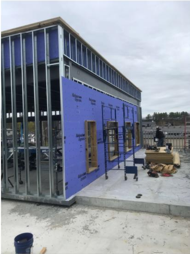
Photo 1: Installation of the gypsum wall and window blocking at the bunker rooms façade.
