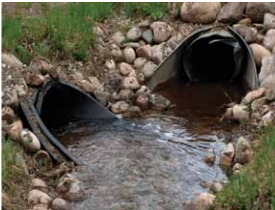
Stormwater leaves the storm drain through an outfall.
